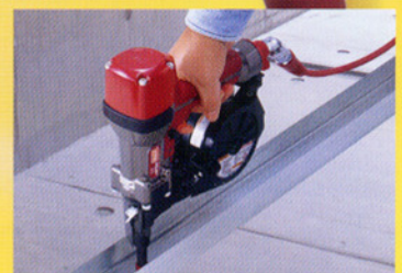
Metal Track to Concrete Ceiling (Ideal Super Light & Compact Tool for Overhead Use)
